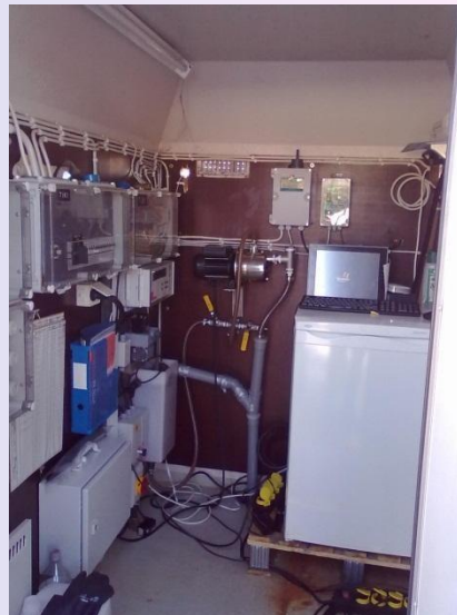
Control System installations
