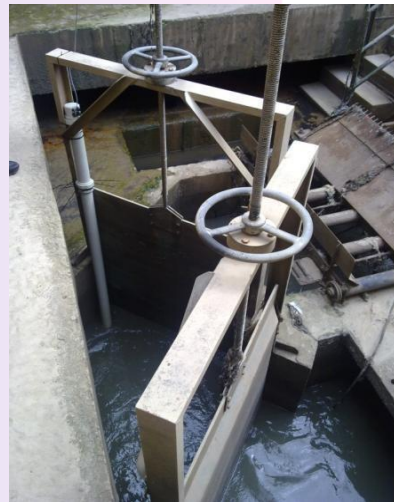
Probe system installed at the pumping station
